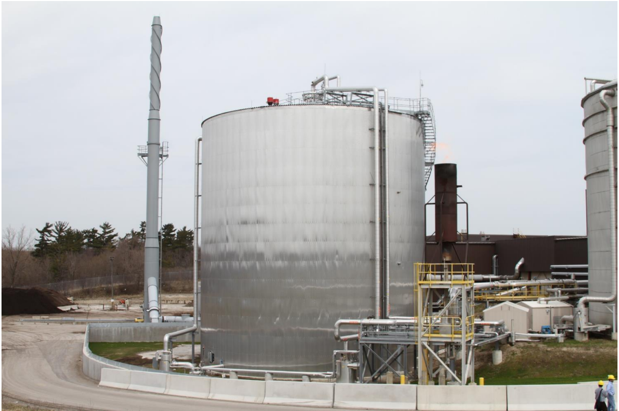
Figure 3. Low Solids Anaerobic Digestion System for SSO in Toronto, Canada
